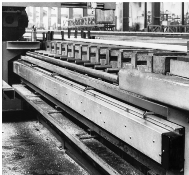
LSVG Powerail feeding a production machine
