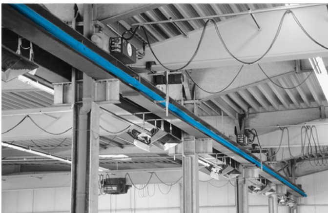
LSV serves for OHT crane electrification
